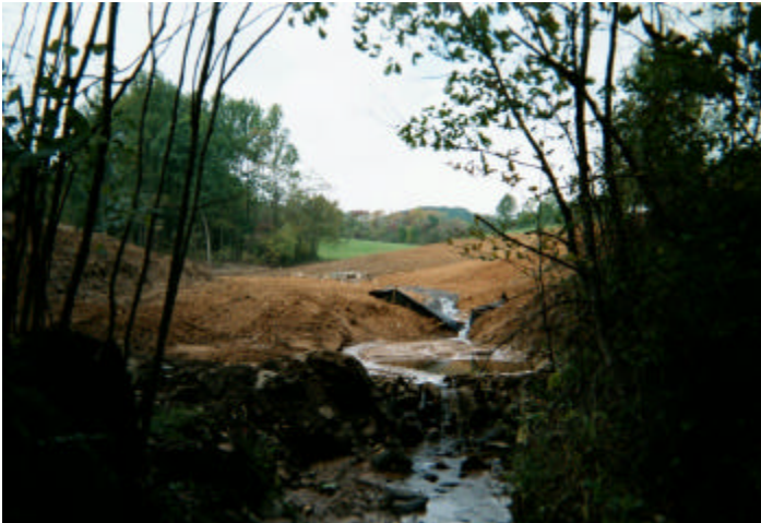
Figure 12. Failing ESC practices at a construction site in Catchment 104
