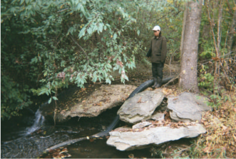
Figure 30. Outfall pipe from a sludge field
