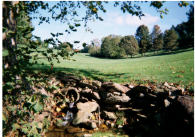
Figure 28. Stream section in need of daylighting
