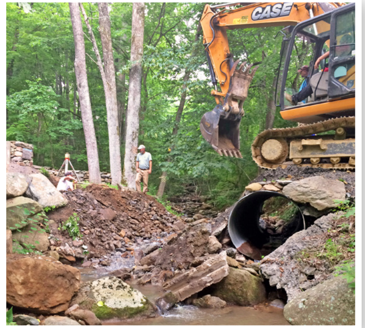
The removal of culverts at Sprucepine Branch in Rappahannock. Photo by Claire Catlett
