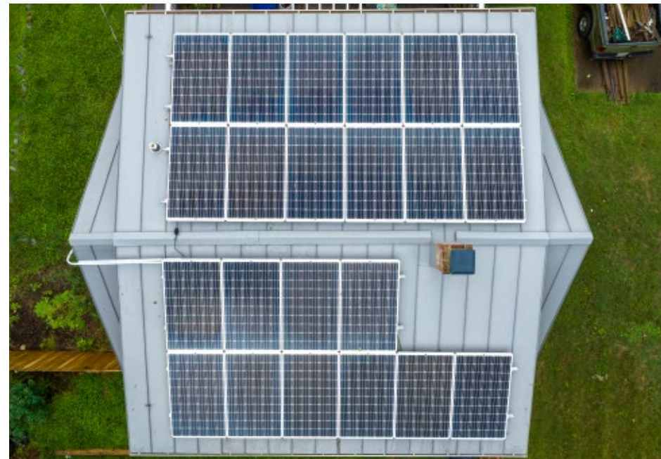
SOLAR PANELS INSTALLED THROUGH SOLARIZE PIEDMONT ON A HOME IN WARRENTON. Photo by Hugh Kenny
